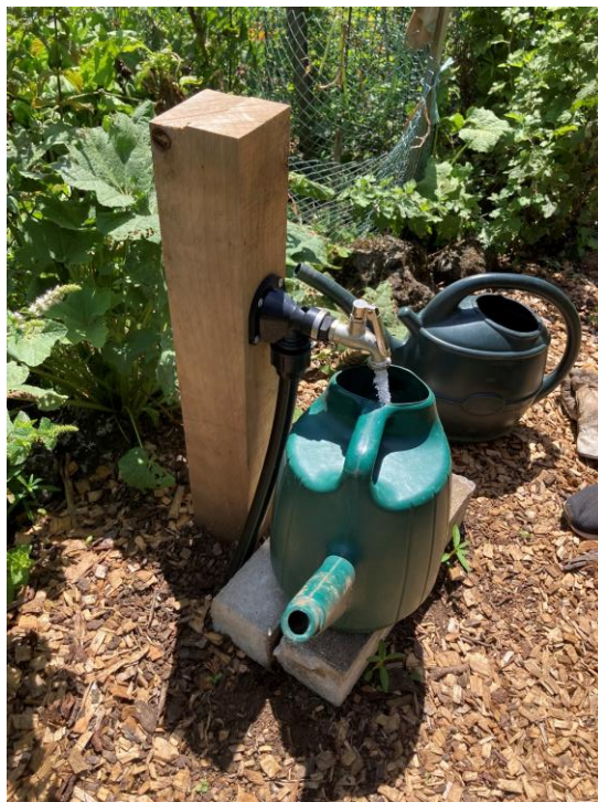
One of the Water Outlets filling a Watering Can.
