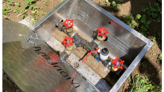
Water Flow Distribution Control System.
