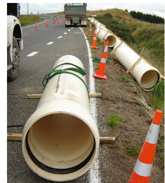
DN575 (630mm OD) PN9 WHITE RHINO for a wastewater outfall, installed under a sealed road, Edendale, Southland.
