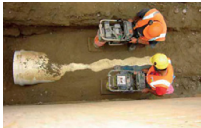
DN600 PVC-U stormwater pipe, showing a deep installation with correct mechanical side compaction of bedding and surround materials in layers, Edendale, Southland.
