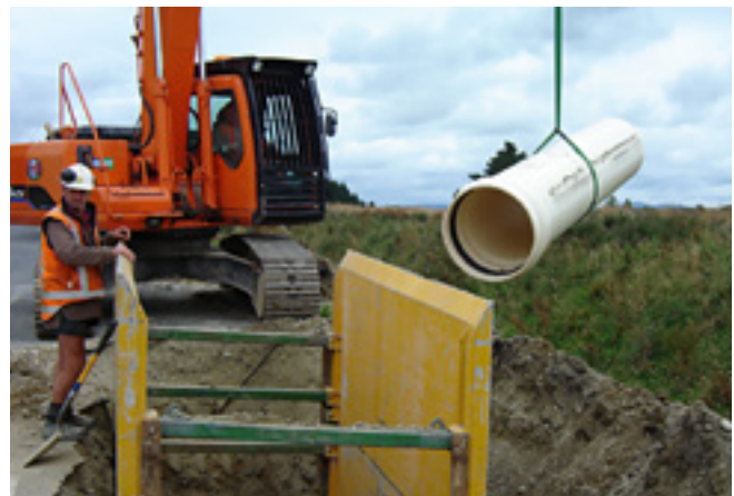
Installation of 3 metre lengths DN600 PVC-U stormwater pipe in trench shields, showing correct lifting with a nylon strop, Edendale, Southland.
