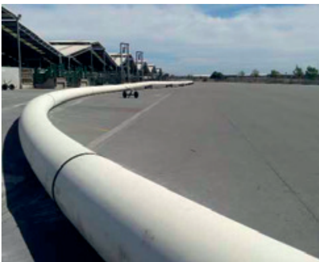
DN710, PN12.5, PE100 sewer rising main being prepared for installation by horizontal directional drilling. Pipe is black with a cream coloured jacket, identifying it visually as a pressure sewer in accordance with AS/NZS 4130, Christchurch City.
