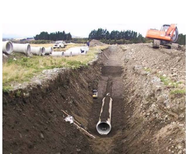
Iplex PVC-U DN450 sewer main installed in Te Anau 2001, to replace a earthquake damaged concrete pipeline, and which has endured all earthquakes in the area since, undamaged.
