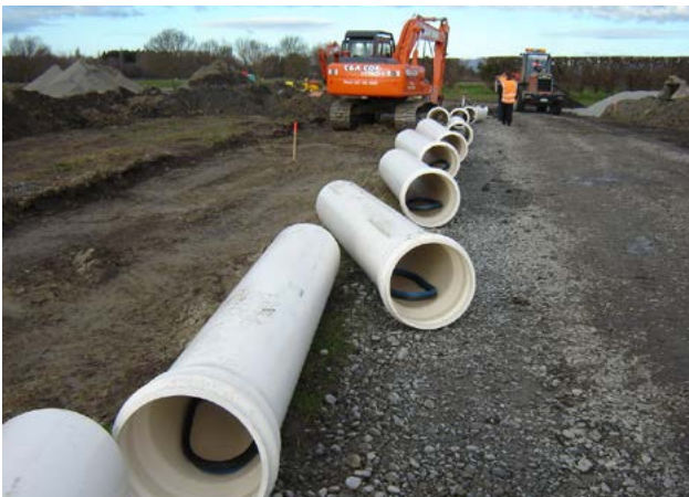
Iplex Novakey® DN450 PVC-U pressure sewer rising main, laid near Belfast, Christchurch in 2005, which endured the 2011 Canterbury earthquake sequences undamaged.
