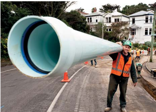
Iplex Apollo® Blue PVC-O DN150 PN16 pressure watermain, installed in Kelburn Parade, Wellington City, in 2011, specifically to improve seismic resilience in the area, which endured the November 2016 Kaikoura / Culverden earthquake sequence, undamaged.
