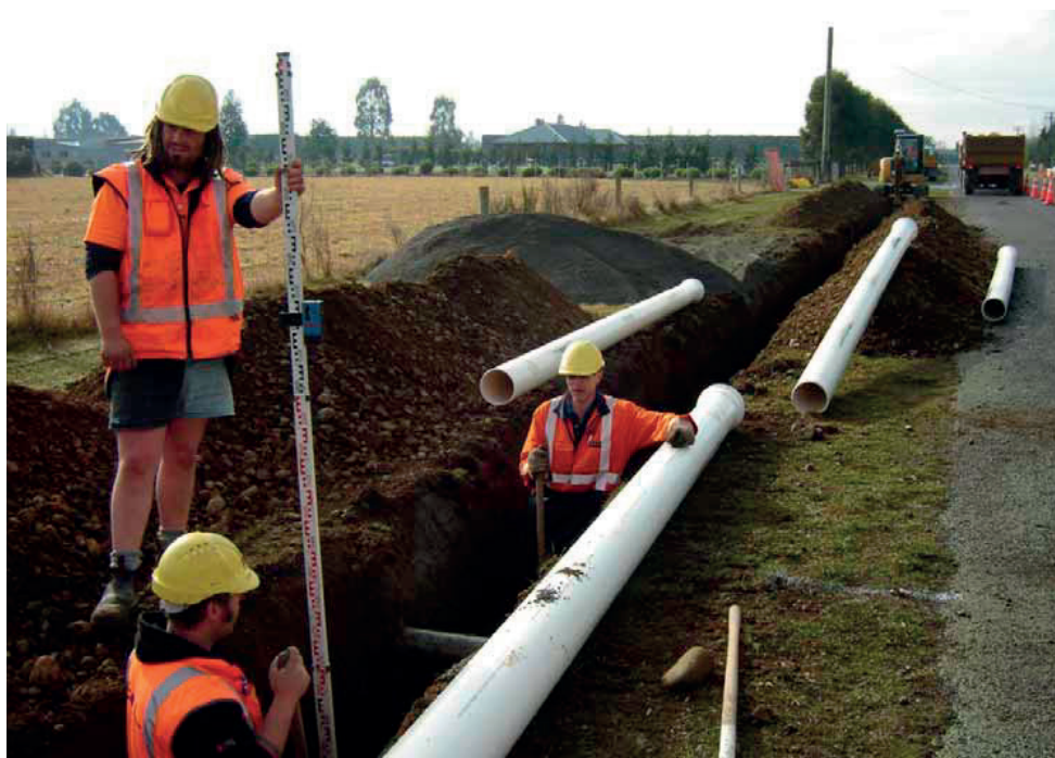
Installation of NOVAKEY™ Series 1 PN 12 pipes, in a road berm near Ashburton, with laser assisted control of the trench depth and grade.
