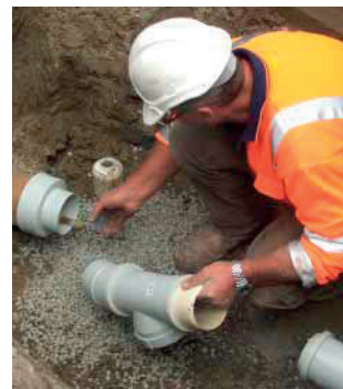
Installing DN100 NOVADRAIN™ pipe with coupling and inspection pipe fitting, Christchurch City.
