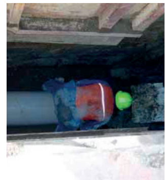
Deep installation of NOVADRAIN™ DN300 SN4 at 4.8m cover under main road, Gisborne City.
