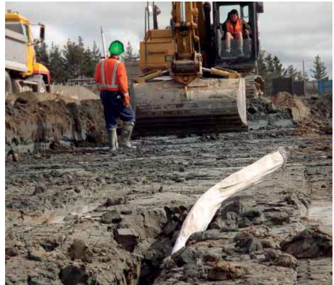
NEXUS™ HI-WAY with factory-fitted filter sock being installed in preparation for the road base, Longburn, Manawatu.
