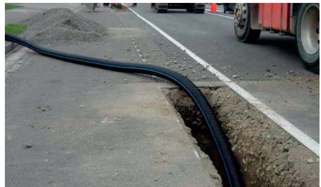
NEXUS™ FLO interceptor drain installation in a lightly loaded section of the highway environment, Tremain Ave, Palmerston North City.
