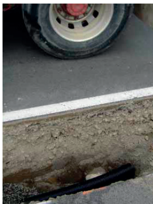
NEXUS™ FLO interceptor drain installation in a lightly loaded section of the highway environment, adjacent to the main wheel loaded zone, Tremain Ave, Palmerston North City.
