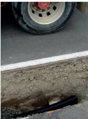
Iplex NEXUSFLO interceptor drain installation under the berm of an arterial commercial/industrial roading environment, Tremaine Avenue, Palmerston North City.
