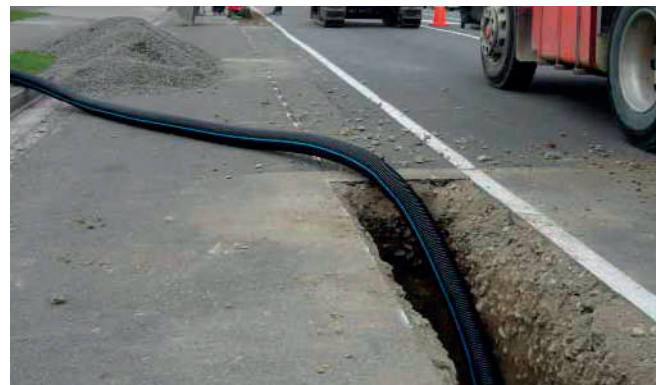
Iplex NEXUSFLO interceptor drain installation under the berm of an arterial commercial/industrial roading environment, Tremaine Avenue, Palmerston North City.
