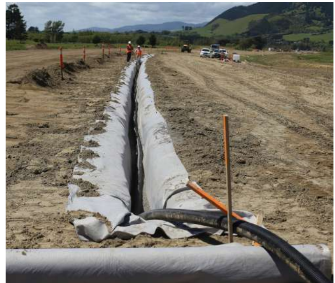
Iplex NEXUS HI-WAY being installed for Expressway road drainage construction, Kapiti Coast
