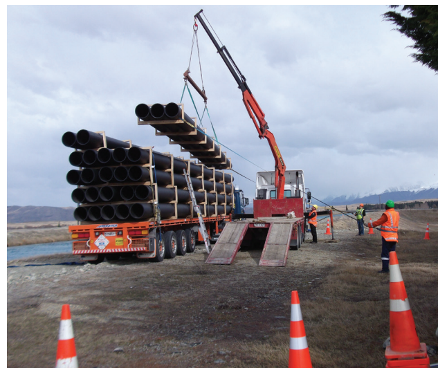
DN500 PN8, PE100 pressure water main pipe lengths in factory transport crates, being unloaded on site, Lake Tekapo Canal, Mackenzie District
