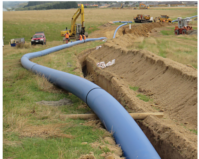
Iplex POLIPEX DN 500 PN PE100 pressure pipe coloured black with blue jacket identifying it as a pressure water mains, Manawatu District.
