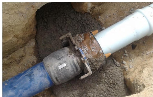
Figure 5.3 - Concrete thrust block with vertical tie bars, supporting an in-line flanged connection between Iplex PVC and PE pressure pipes at a river crossing, Waitaki District
