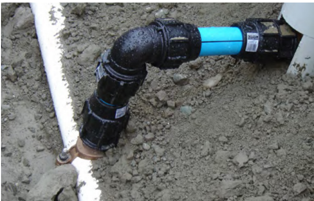
Figure 3.12 - Gunmetal tapping saddle with a male threaded adapter on white DN100 Series 1 Iplex® PVC water main, connecting to a DN50 Iplex BlueLine® PE service lateral, and valve box, near Wanaka, Queenstown Lakes District
