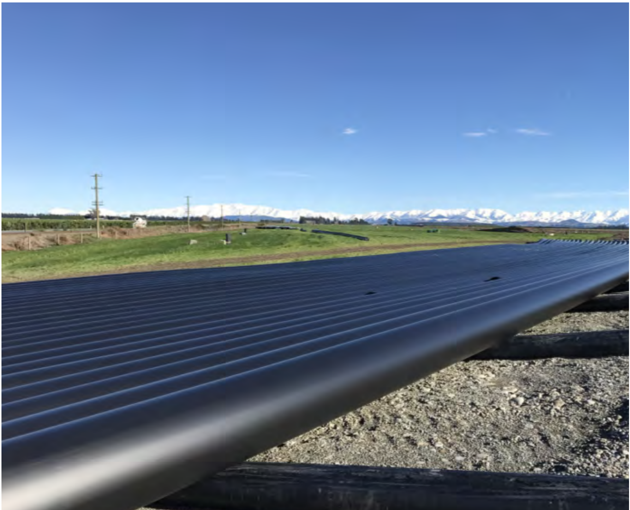
Iplex® PE 100 pressure pipe extruded on site in the Central Plains, Canterbury District.
