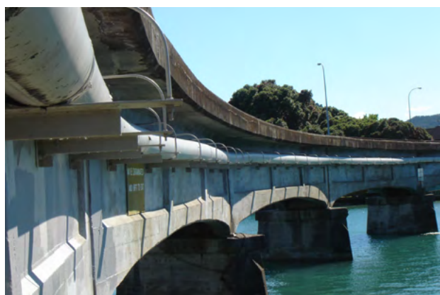
Support brackets for PoliplEx® PE 100 pressure sewer transmission main, including allowance for expansion and contraction, Gisborne City.
