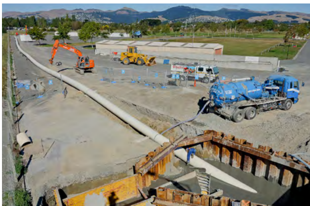
Iplex Poliplex® PE 100 pressure sewer transmission main, installed by Horizontal Directional Drilling, Christchurch City.
