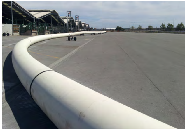
Iplex Poliplex® DN710, PN12.5, PE 100 sewer rising main being prepared for installation by horizontal directional drilling, in Christchurch City. Pipe is black with a cream coloured jacket, identifying it visually as a pressure sewer in accordance with AS/NZS 4130.
