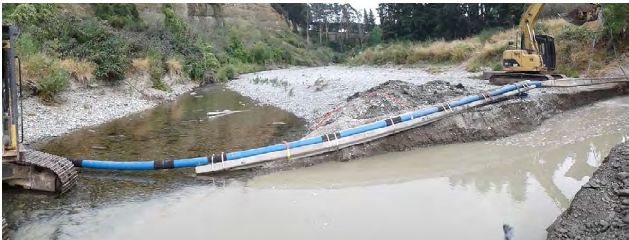
Iplex Poliplex® PE 100 pipe, installed in a river crossing, for a drinking water transmission main, Waitaki District.
