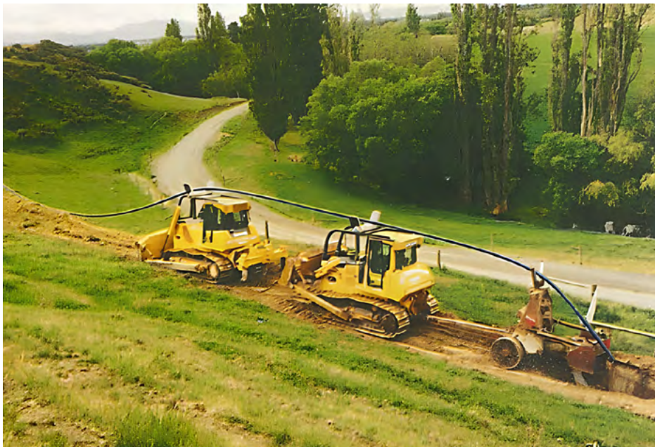
Iplex Blackline™ PE 100 pipe installation by mole ploughing, for stock drinking water supply.
