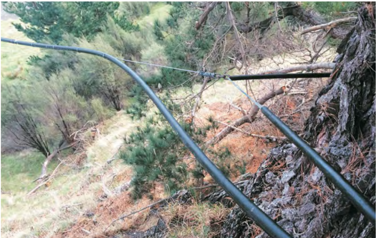
Iplex Blackline™ HP PE 100 pipe, installed in an aerial river valley crossing for stock water supply, Pohangina Valley, Manawatu District.
