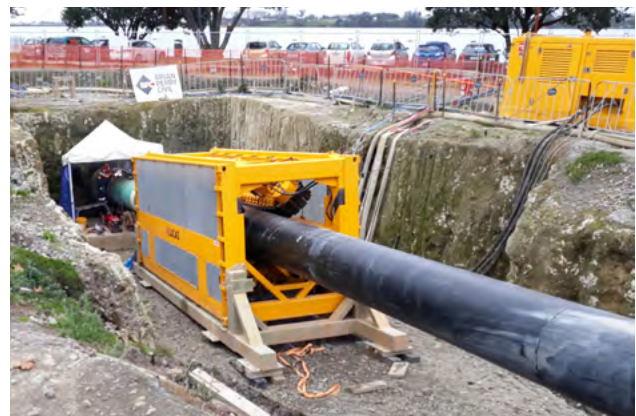
Iplex Poliplex® PE 100 pressure sewer transmission main, installed by Slip Lining, Tauranga City.
