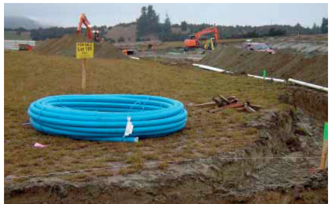
Coil of DN 63 PN 12.5 BlueLine polyethylene pipe on site, near Lake Wanaka.
