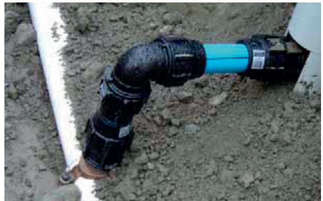
BlueLine pipe and Plasson Line 7 compression fittings used for a water service connection off a PVC-O main to a residential property near Wanaka.
