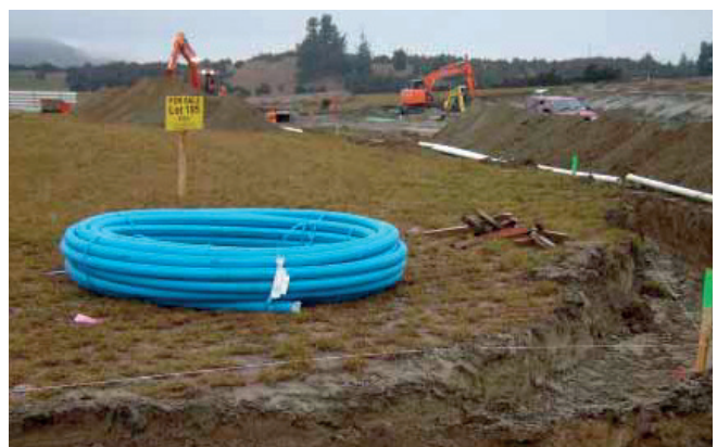
Coil of DN 63 PN 12.5 BlueLine polyethylene pipe on site, near Lake Wanaka.
