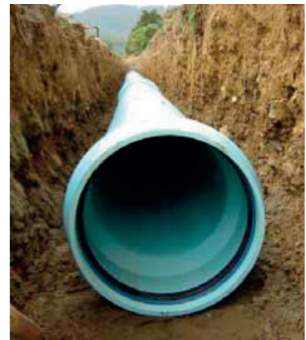
DN450 PN12 BLUE RHINO™ in trench ready for backfilling, under sealed road near Levin.
