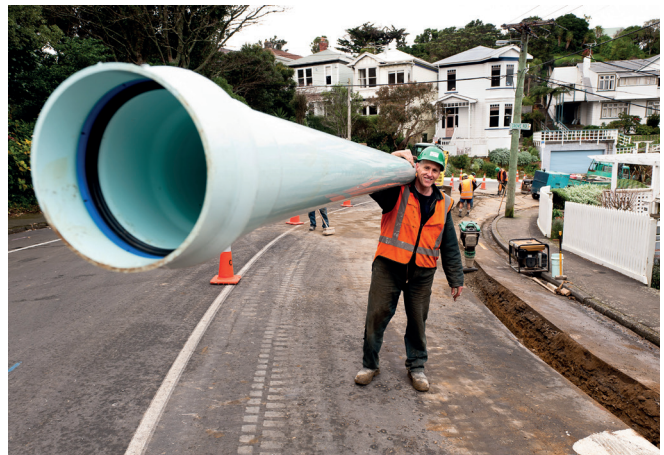
Manual site handling of DN 150 S2 PN 16 Apollo Blue pipe, Wellington City
