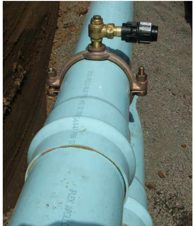
Figure 4.13 - Gunmetal tapping saddle and Under Pressure Tapping ferrule with a Plasson "line 7" male threaded adapter, for an air release point, on a twin DN150 Series 2 PN16 Iplex® PVC pipe, near Oakura, Taranaki District
