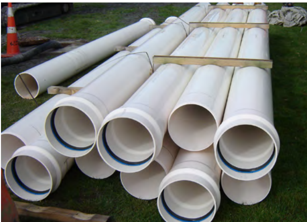
Iplex Apollo® PVC-O DN200 PN12.5, pressure sewer main, installed in Charles St, Kaiapoi, October 2010, which endured the February 2011 Christchurch Earthquake sequence, and all following aftershocks undamaged.
