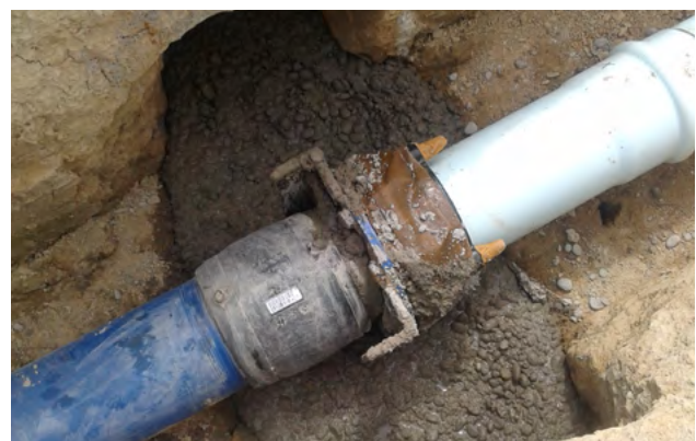
Figure 6.3 - Concrete thrust block with vertical tie bars, supporting an in-line flanged connection between Iplex Apollo® PVC-O and PE pressure pipe at a river crossing, Waitaki District
