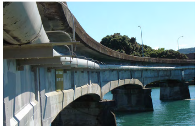
Support brackets for Poliplex® PE 100 pressure sewer transmission main, including allowance for expansion and contraction, Gisborne City.
