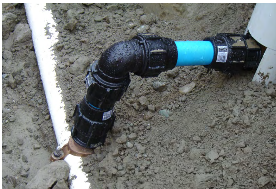
Iplex BlueLine® PE 80 pipe in a drinking water service lateral connection, used with Plasson® Line 7 mechanical fittings.
