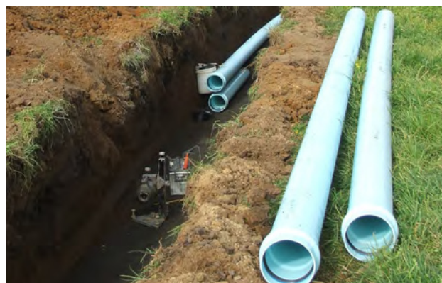
Figure 4.5 - DN150 S2 Iplex PVC pipe used for a pressure sewer rising main - New Plymouth City, Taranaki
